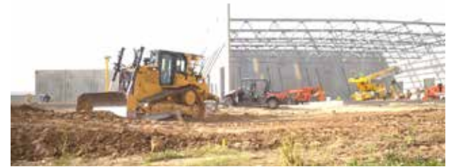
Construction on the new Cereal Ingredients Facility in Eastowne Business Park began in 2021.
